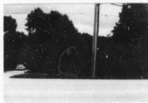
Kauffman Substation - York Road - front view from opposite side of road
