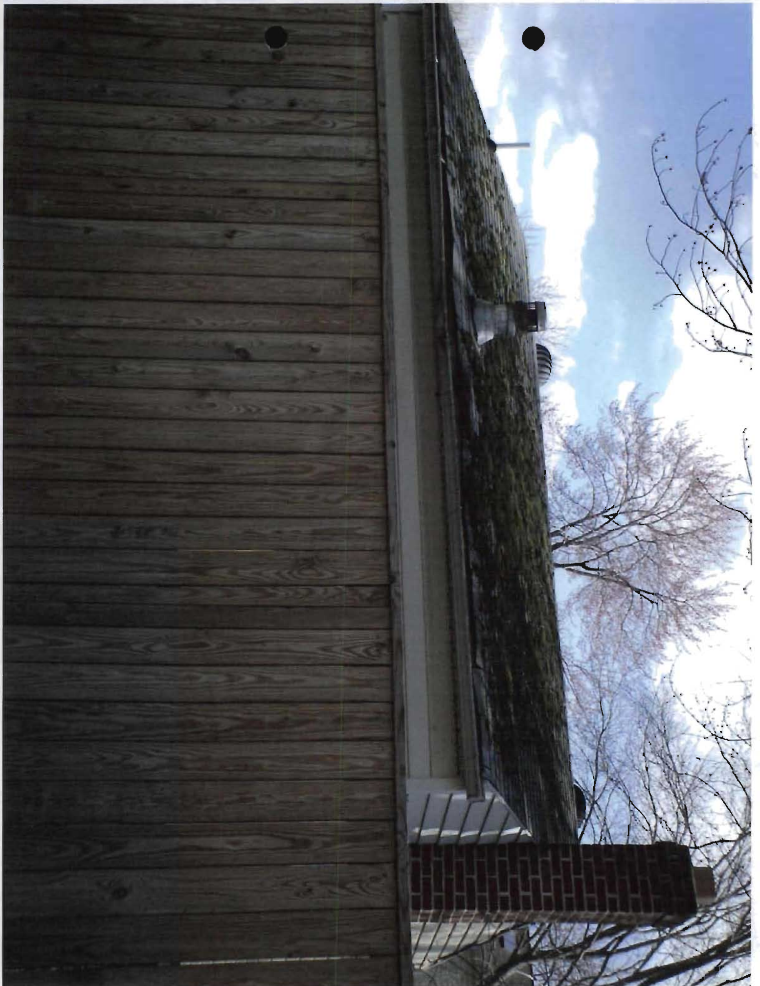
View of Protestor's shed with moss on roof
