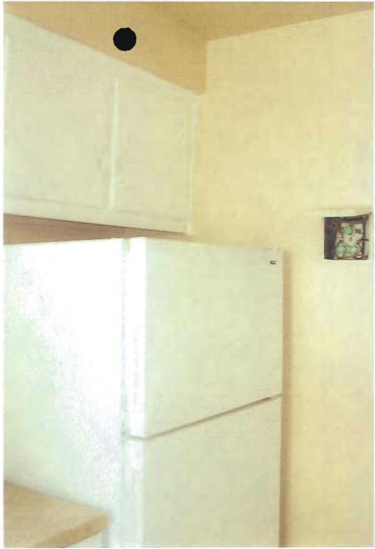
2nd Floor Kitchen Apt. (fuse box)
