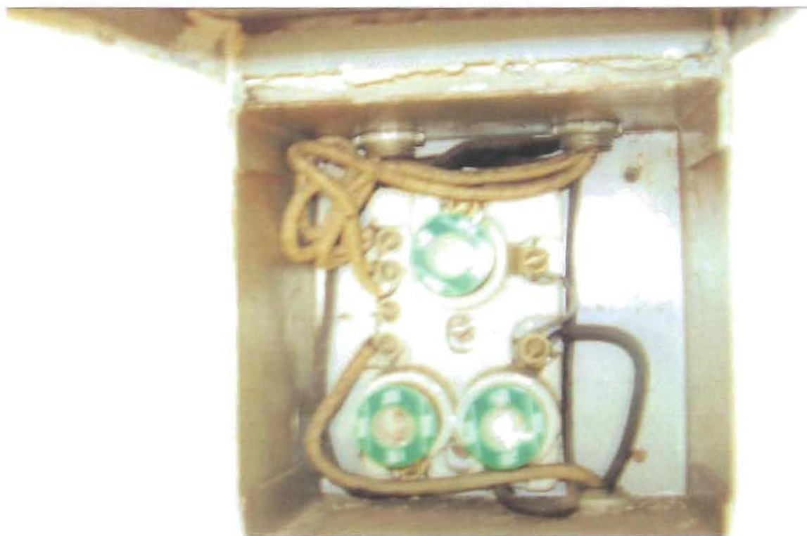
1st Floor Kitchen Apt. (fuse box)
