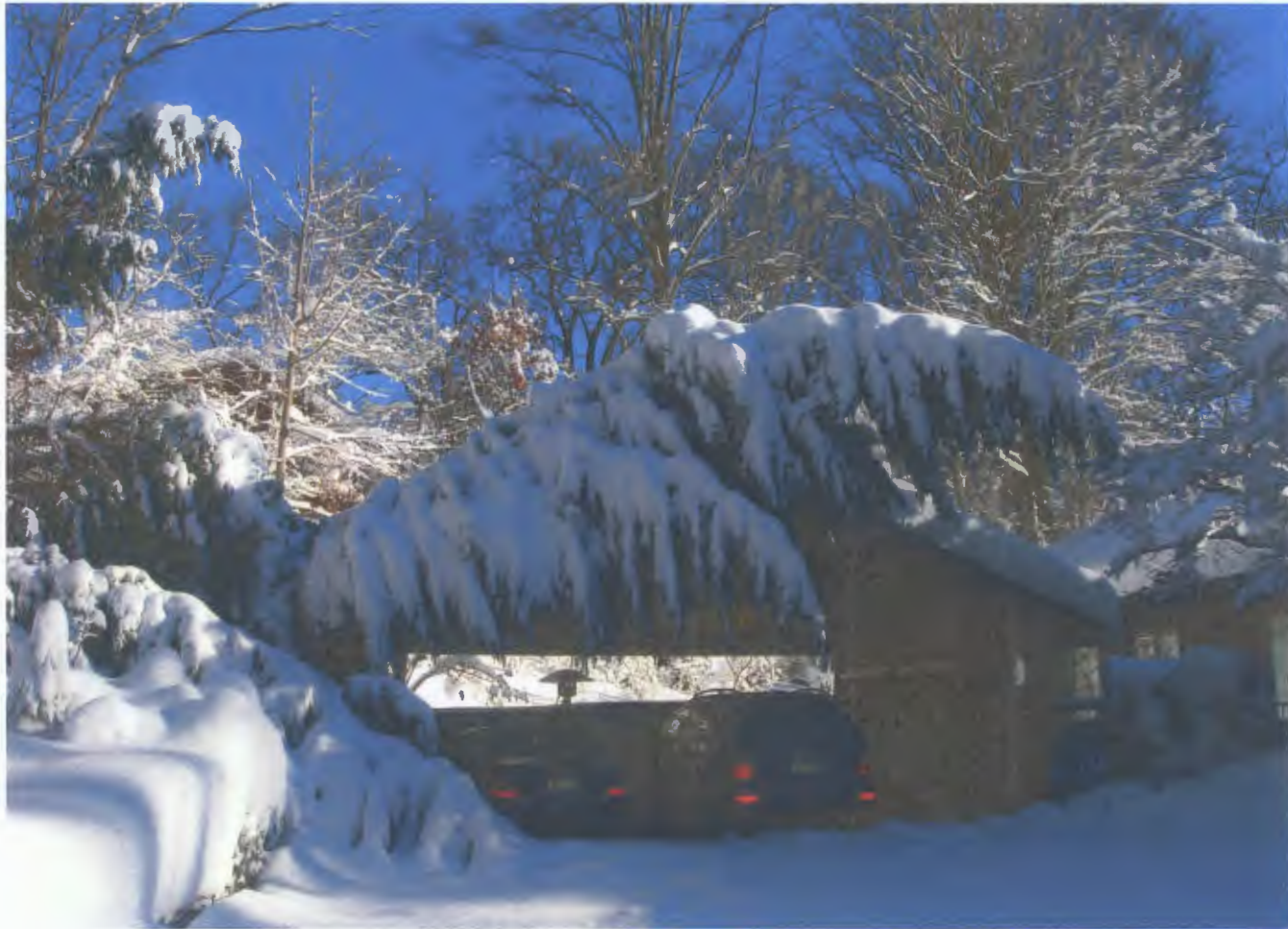
PRIOR CARPORT, SAME SITE, DAMAGED IN SNOWSTORMS BY FALLEN TREES.
