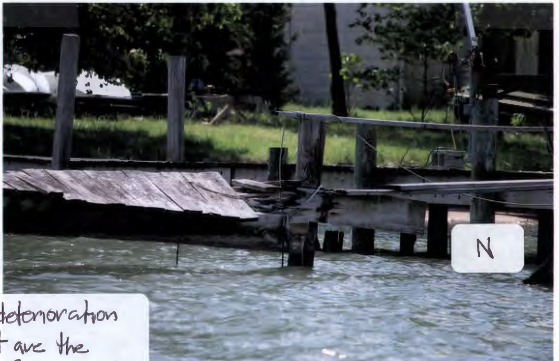
Parts of "pontoon lifts" (this one inoperable) are strewn about the property
