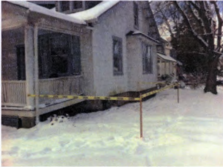
The 9ft porch roped off.
