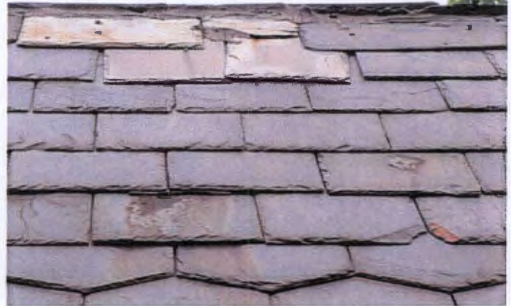
Slate roof in need of repair work.
