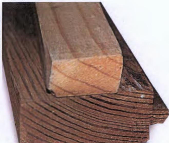
Historic windows are made of old growth wood which is superior to wood products available today. It is denser and prevents insect damage and water penetration better than new growth wood.
