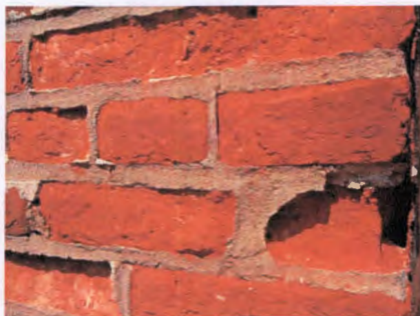
Aggressive cleaning methods probably contributed to the erosion of this brick facade.
