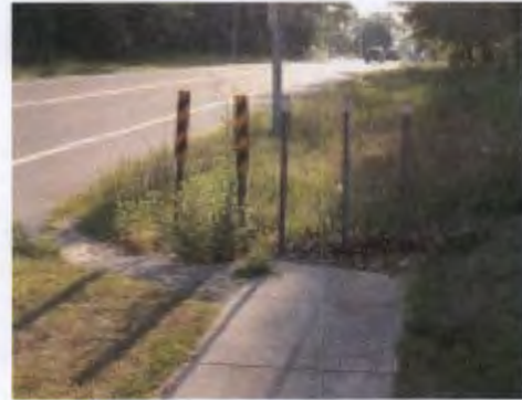
A sidewalk gap on Ebenezer Road
