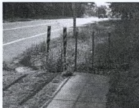
A sidewalk gap on Ebenezer Road
