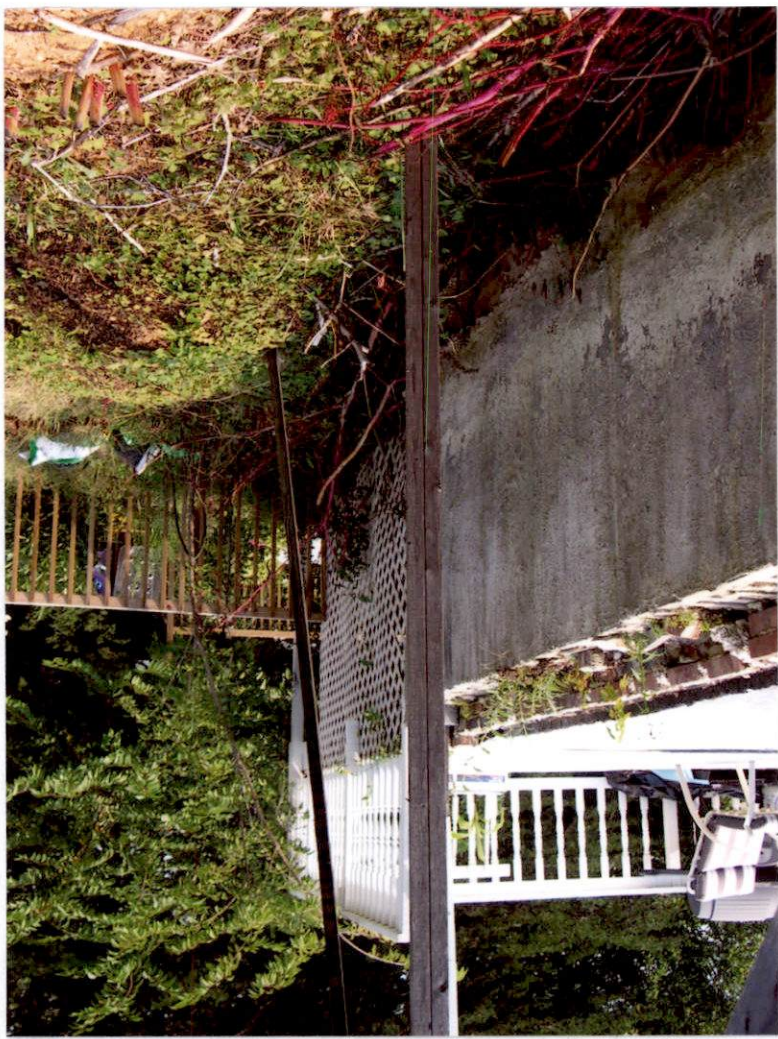
Brick Planter is on Car port is gone. Showing exposed block wall.
