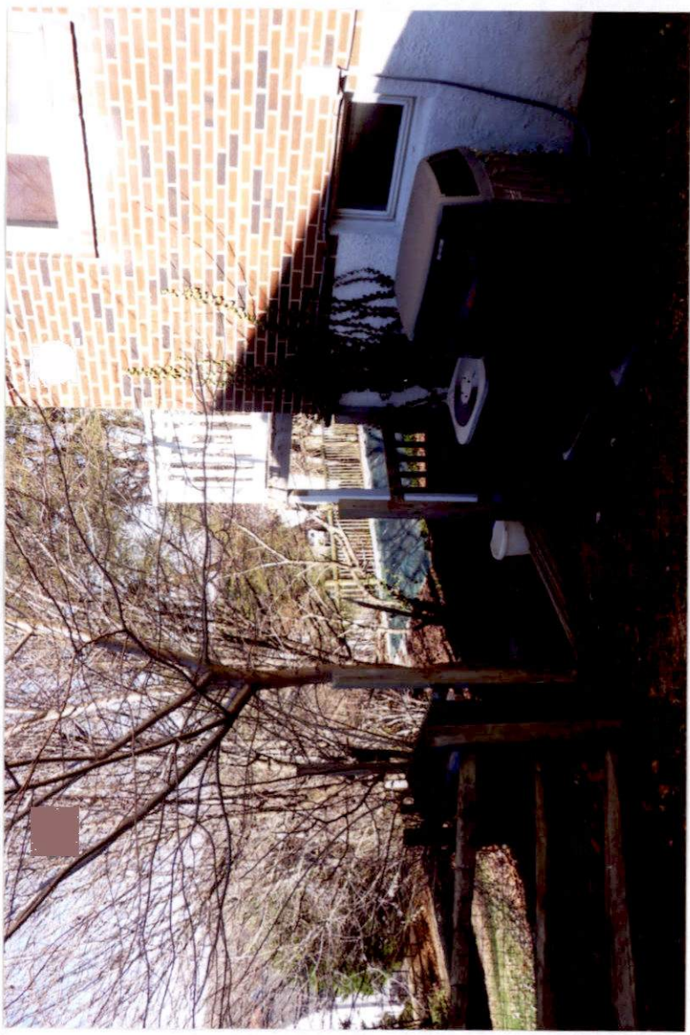
Photos Taken June 2016 Pool Broken gate fence gate
