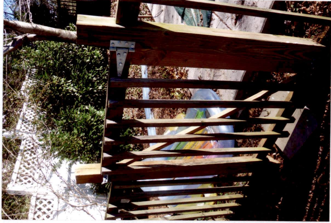
Pool Back gate closing Fence self closing is not
