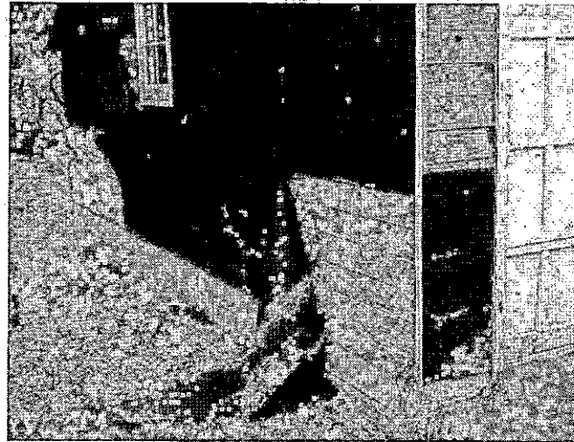
Garage front left damage and garage door cracked
