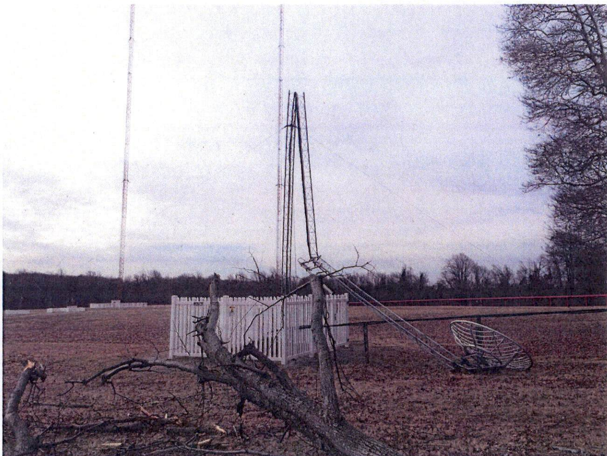
Photo 4 of 4 (damaged in storm April 2015)
