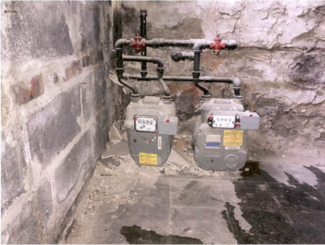
Twin gas meters with galvanized pipe
