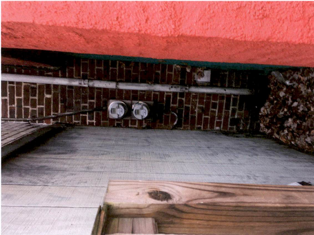
Twin electric meters
