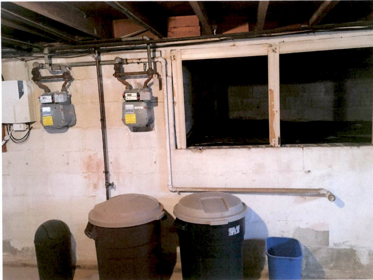
Multiple gas mains with original steel piping
