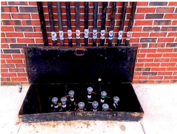
Secure Bulk Tank Fill Pipes and Catch Basin
