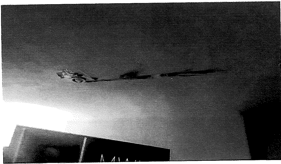
This photo shows the deteriorating roof, severely leaking during a mild rain.
