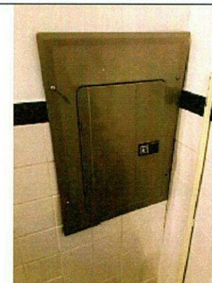
Safety Item # 18 System : Electrical Location : in law bathroom
