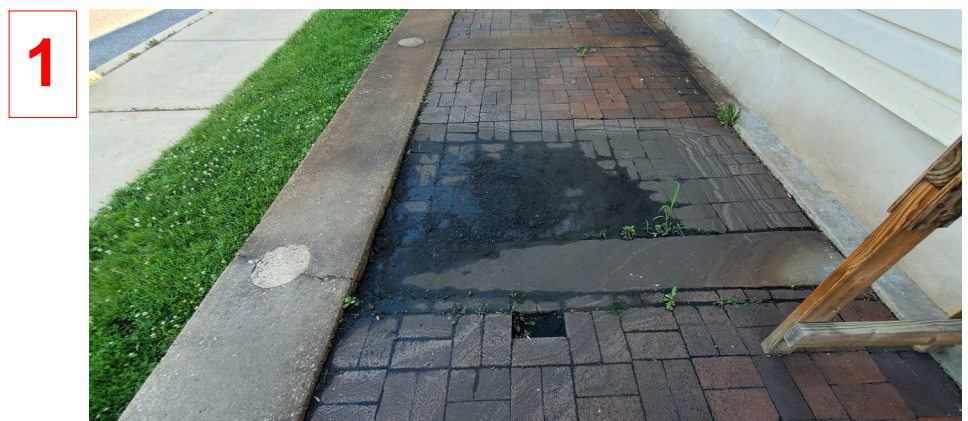
NOTE: PURPOSE OF THE PHOTOGRAPH IS TO SHOW THE EXISTING WALKWAY CONDITION FOR REPAIR
