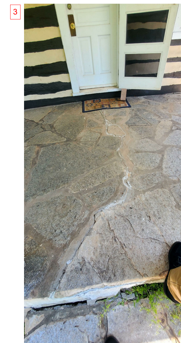
NOTE: PURPOSE OF THE IMAGES IS TO AID IN THE DOCUMENTATION OF EXISTING CONDITIONS IN ADDITION TO PROVIDING CONTEXTUAL VISUAL INFORMATION FOR REPAIR
